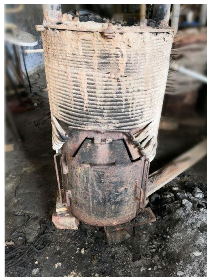
Fig. 3 Photographic view of the Furnace
